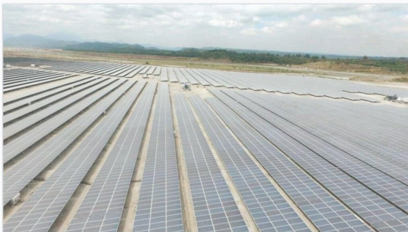
PV Panel Arrangement On-site
